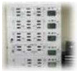
Refrigeration control machine
