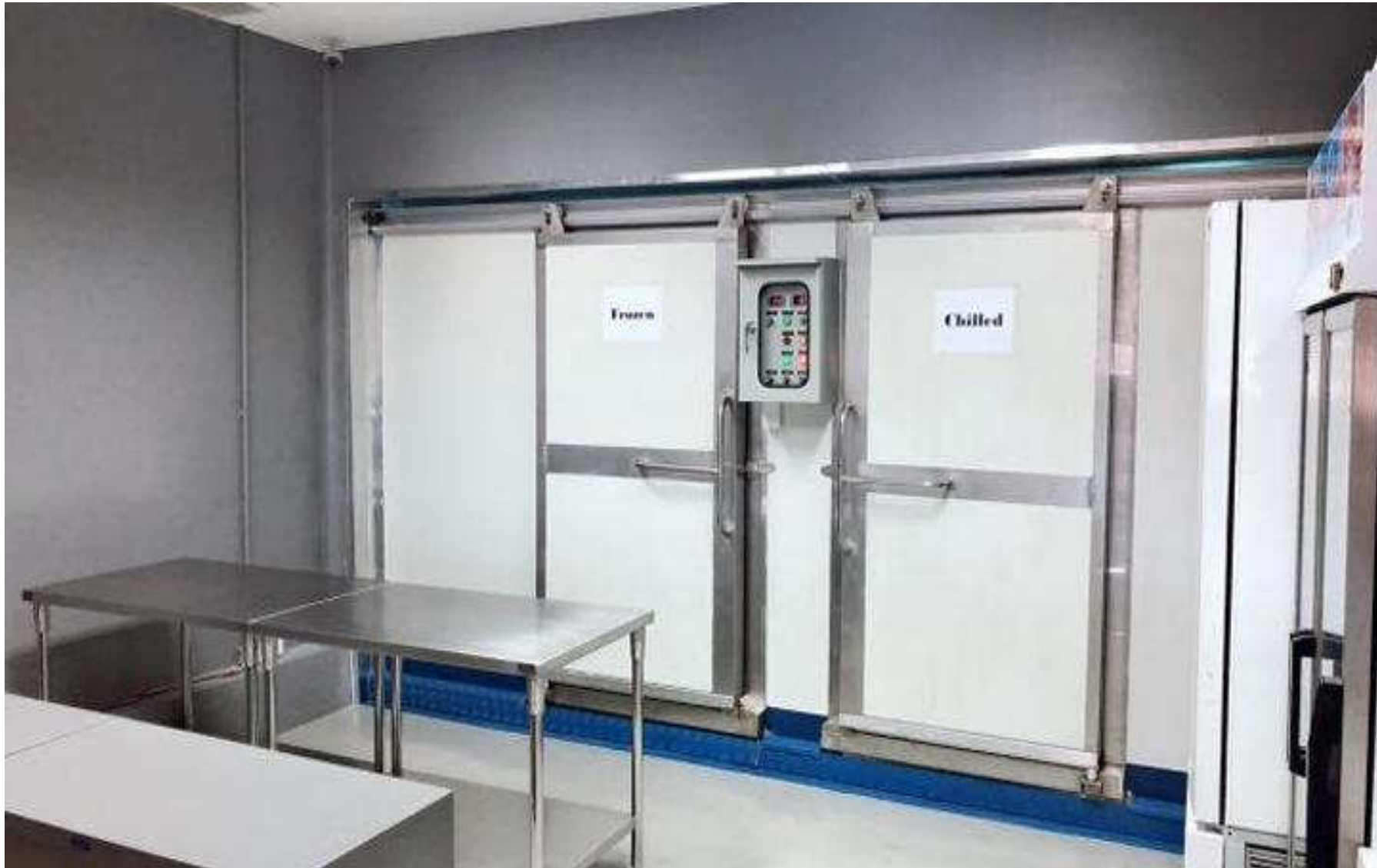
Packing and Temperature Controlled Storage
